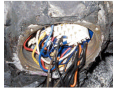
Post Fire Inspection
